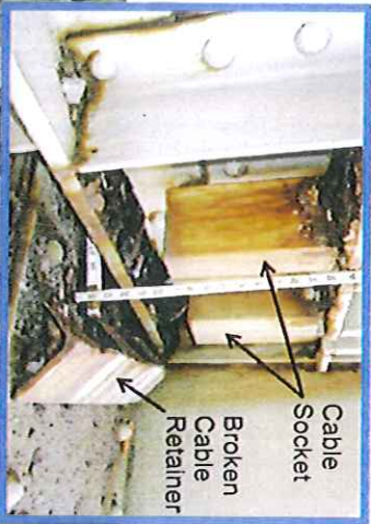
Replace all Cable Retainers
